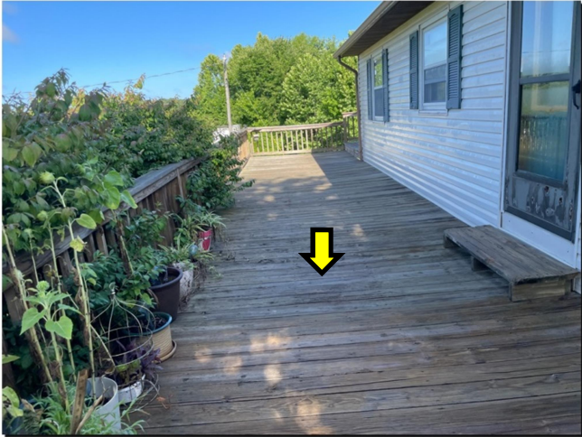
Photo 1 – Deck surface sagging
