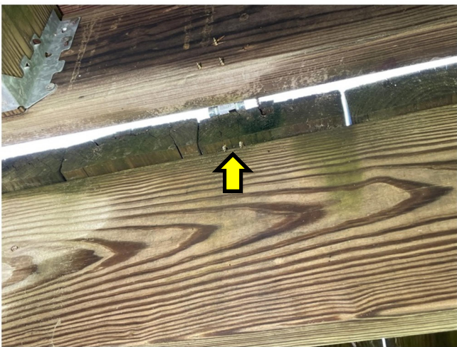
Photo 11 – Weak screw connection
