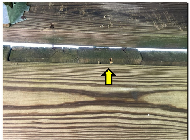
Photo 12 – Weak screw connection
