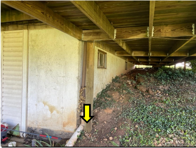
Photo 7 – Support post has settled
