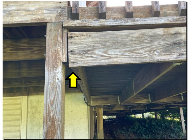
Photo 10 – Inadequate beam support
