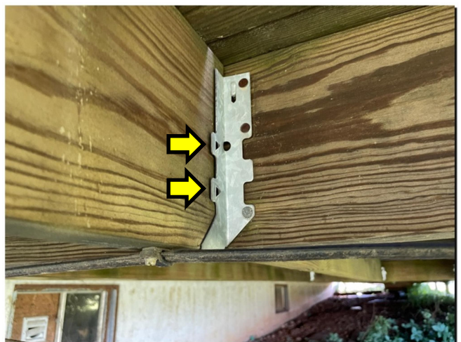
Photo 6 – Missing joist hanger nails
