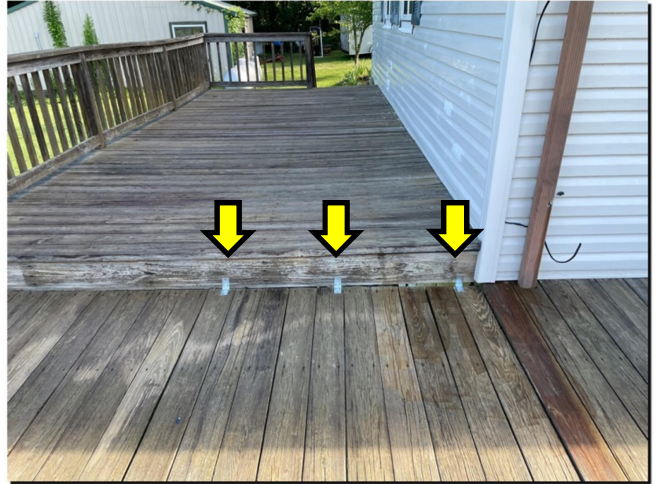
Photo 2 – Recent attempt to repair
