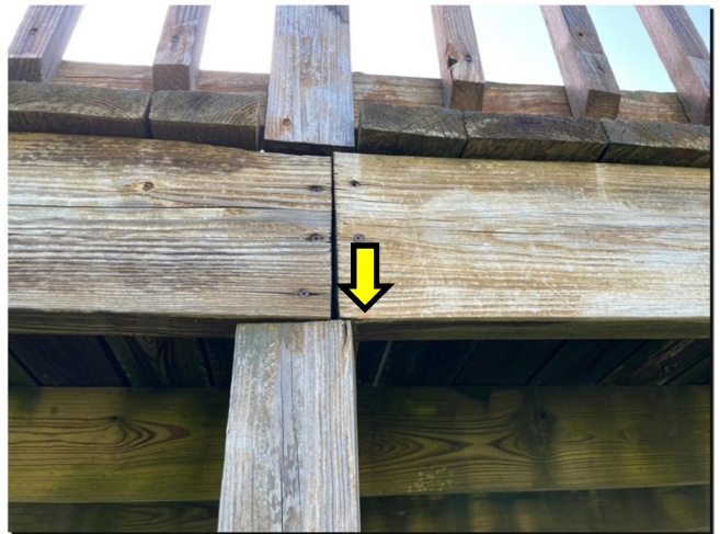
Photo 4 – Inadequate beam support
