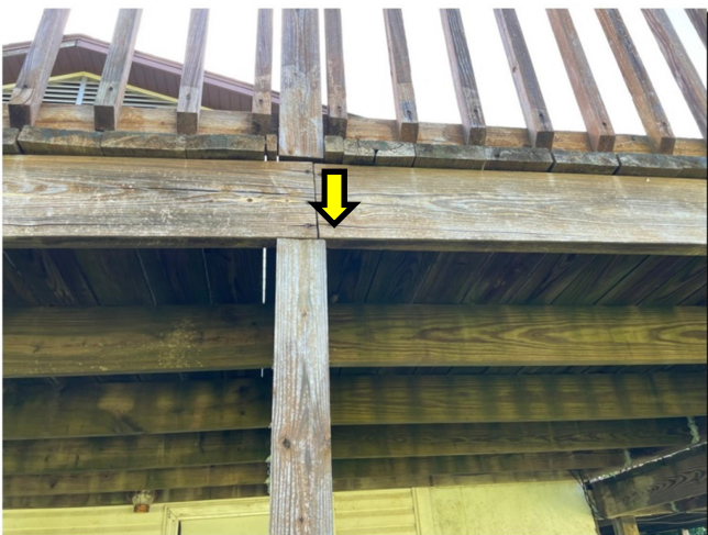
Photo 5 – Inadequate beam support
