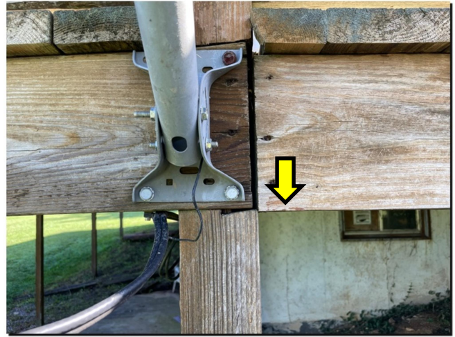
Photo 8 – Inadequate beam support
